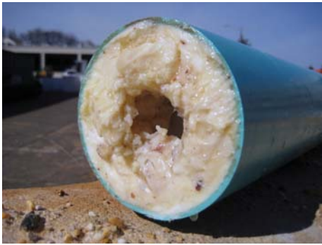
Pipe clogged with fats, oils and grease.
