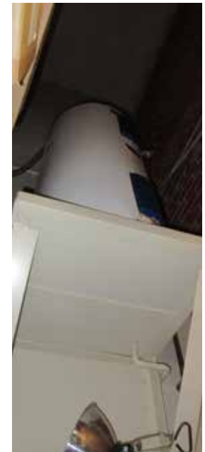
Figure 1-12: Hot water tank within electrical closet
