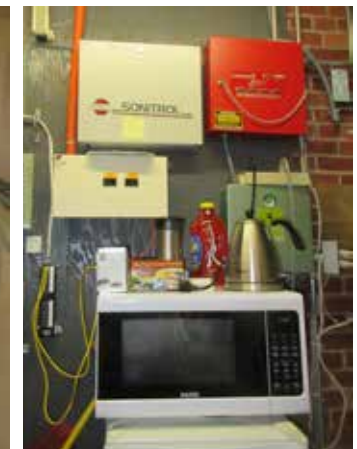
Figure 1-10: Breakroom within sensitive electronic equip.
