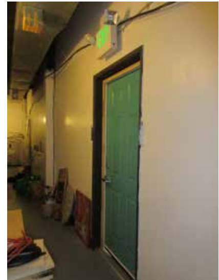
Figure 1-15: Booth Kelly egress exit showing improper egress lighting location and improper exit door hardware.
