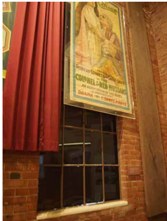
▲ Figure 3: The large “Colonel of the Red Hussars” movie poster hung in a blacked out window which is radiating excessive amount of heat and likely causing damage to the object.
