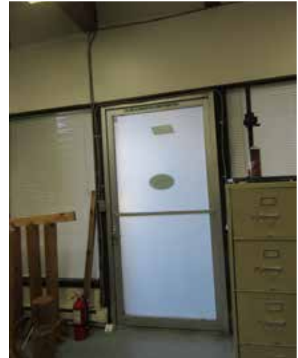
Figure 1-14: Booth Kelly entry. No emergency egress hardware.
