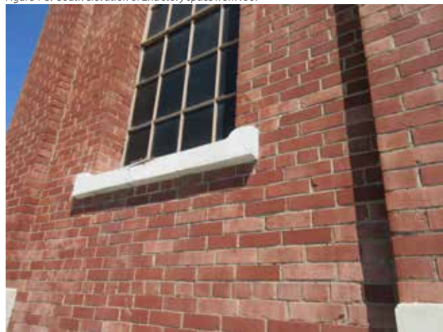
Figure 1-6: Spalling concrete at window sill
